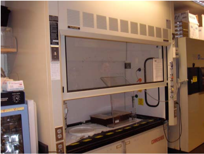
PES hood prior to retrofit with hose that would not allow sash to close
