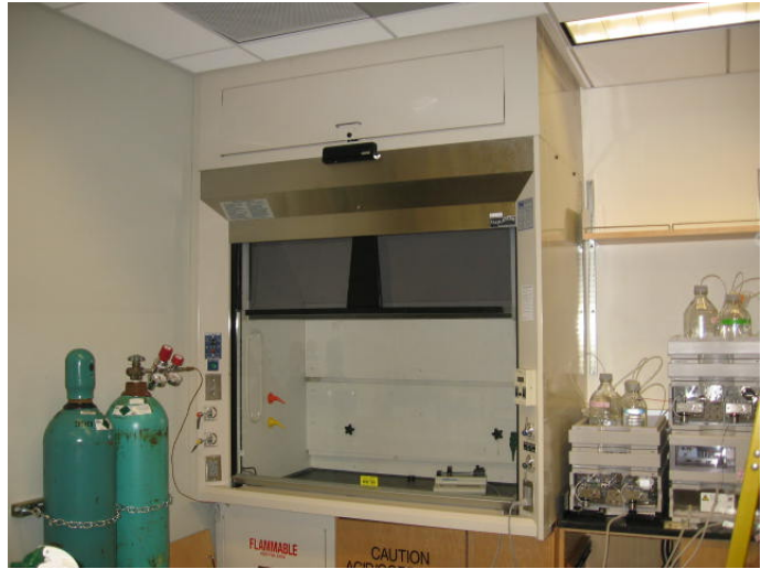
Demonstration Fume Hood in Genome Building Lab 1010
