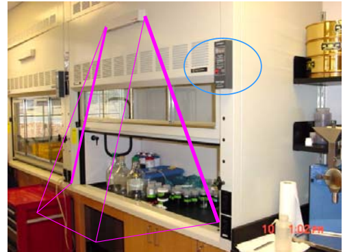
Auto-closure fume hoods with occupancy detection
