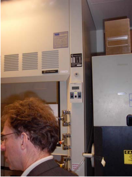
Existing PES hood with VAV control (indicating 105 fpm)
